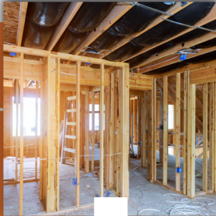
2008- A dramatic, two year, tenants-in-place gut renovation was completed that created 54 efficiency apartments for women.
